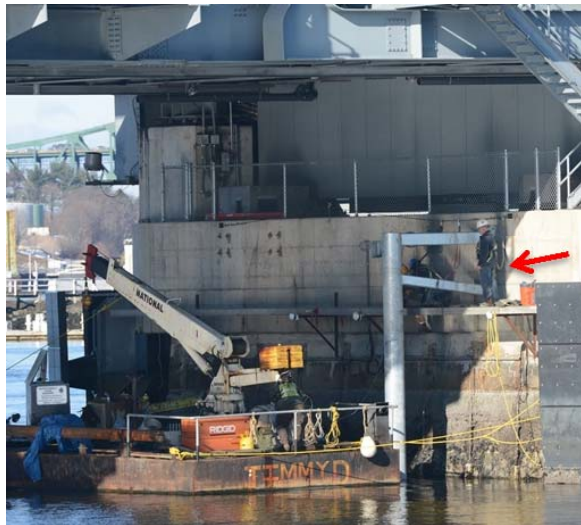
FIGURE 4. INSTALLATION OF VERTICAL GUIDE POSTS (VGP) AT MEMORIAL BRIDGE. NOTE THE INSTALLATION PERSONNEL FOR SCALE (DEC 2016).
